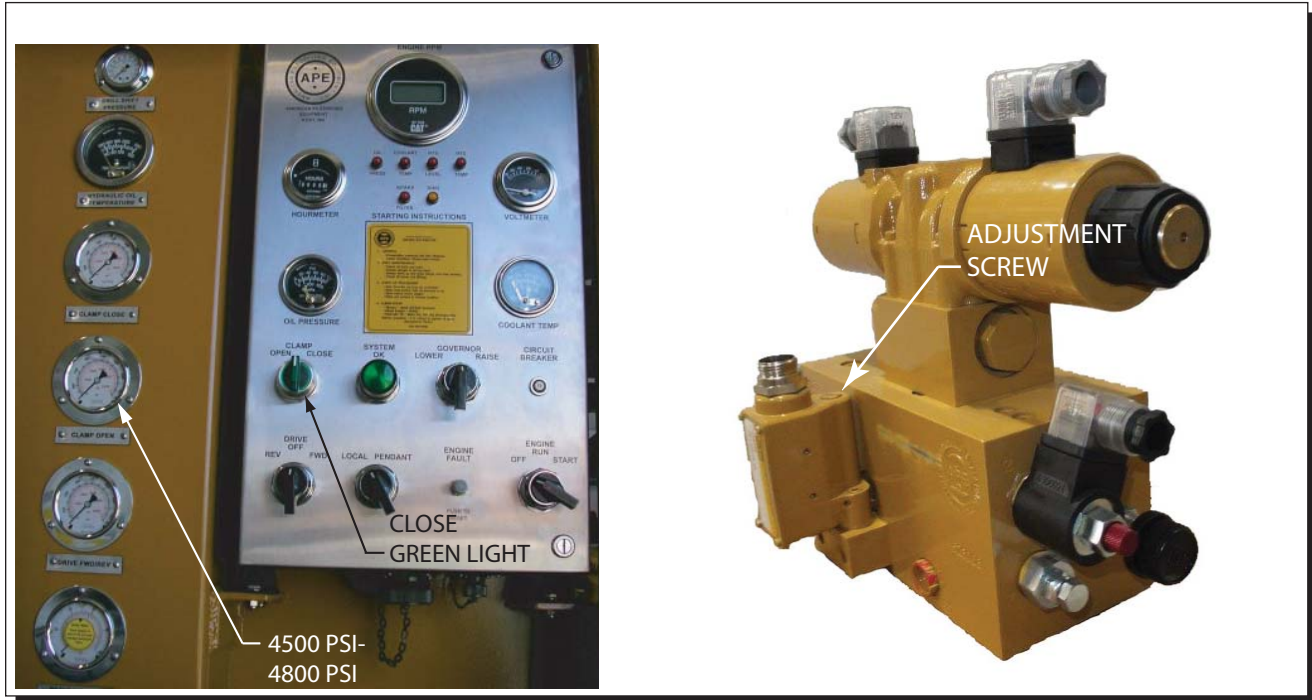
Figure 4-D. Checking Clamp Pressure Switch Setting
