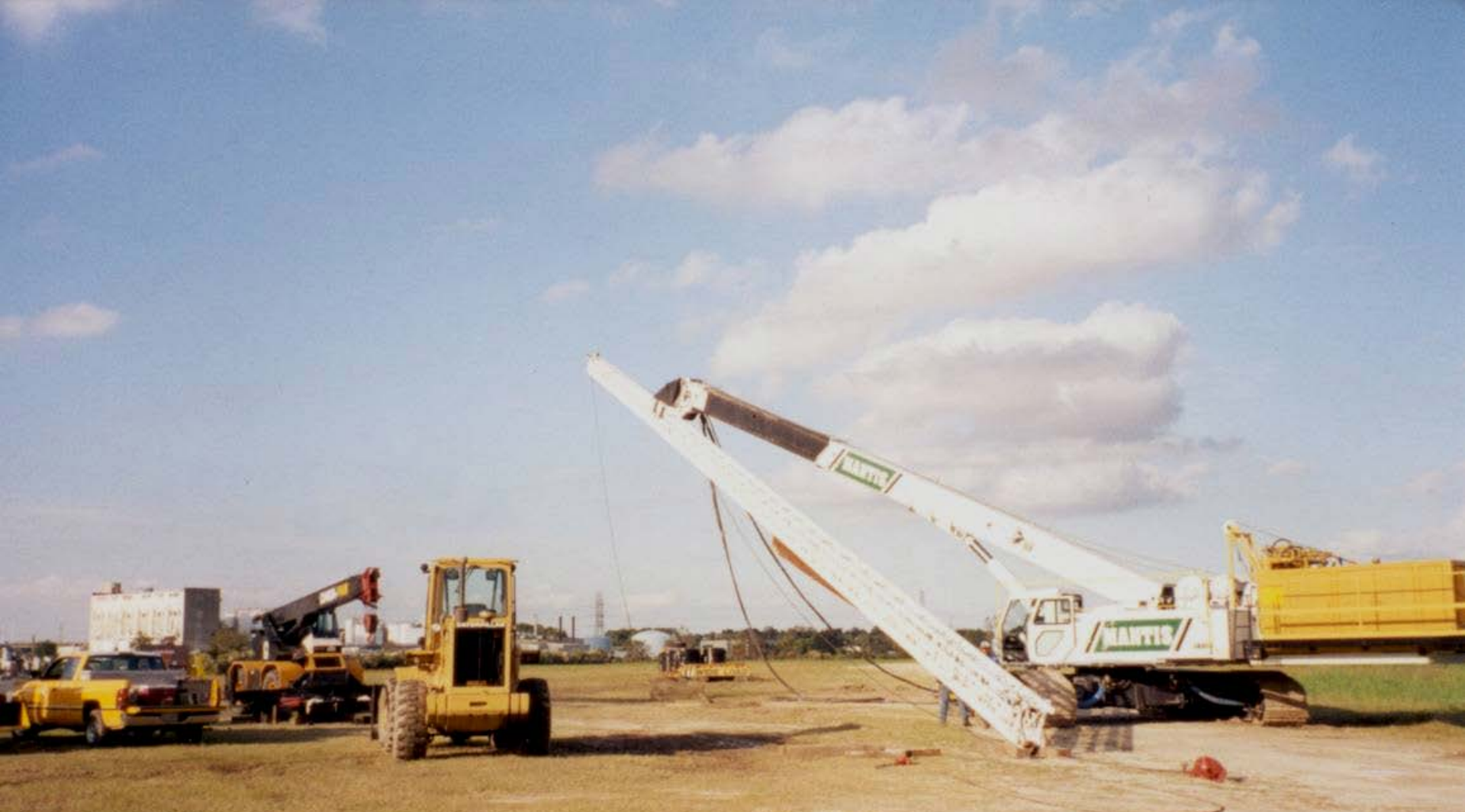
160 feet APE wick drain leads being stood up at Craney Island August 2000. Note: self erecting – no help from other crane.
